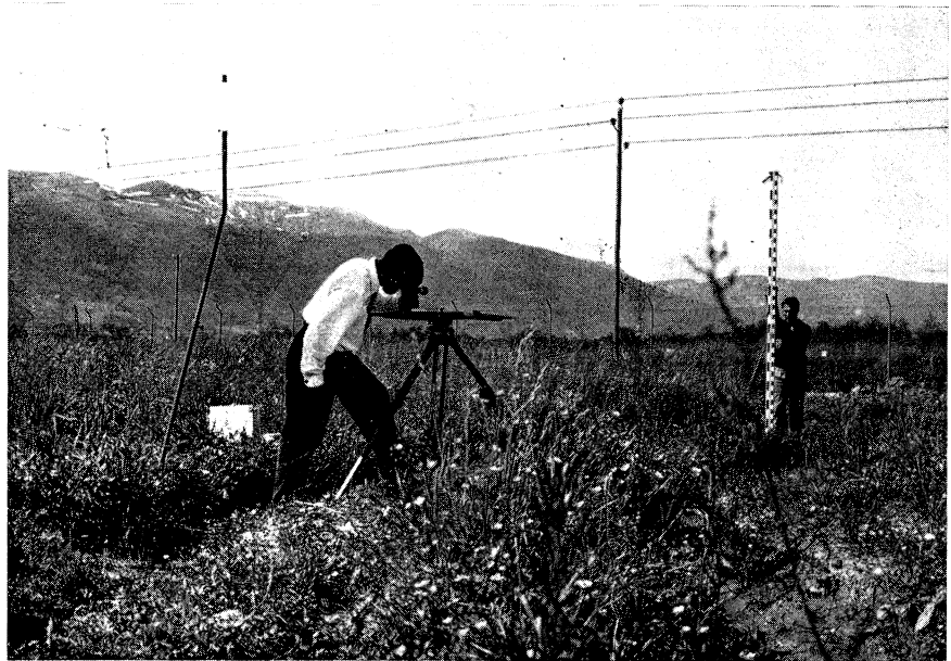
Survey measurements being taken on the ISR site at the end of May. The sunshade was an essential part of the equipment in the intense heat.
